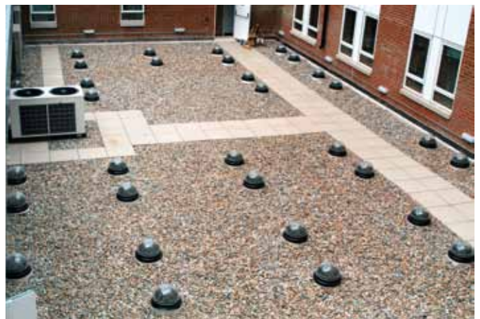
Lewisham Police Station, London, where 50 No. 330mm diameter SunPipes were installed to the cells of this high security building. The SunPipe systems were fitted with vandal resistant top domes and security bars. Stainless steel ceiling trims were fitted with security screws.
